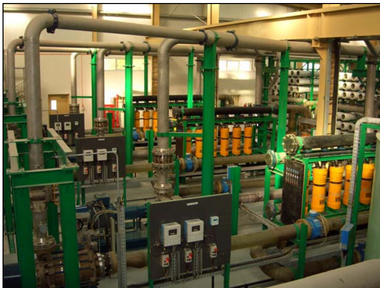
Figure 2 – New Qidfa Plant Overview
