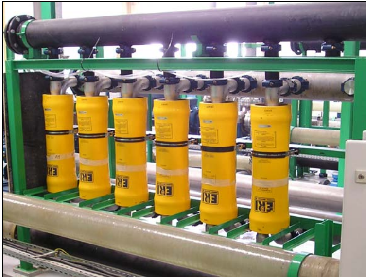
Figure 3 – PX Energy Recovery Device Array
