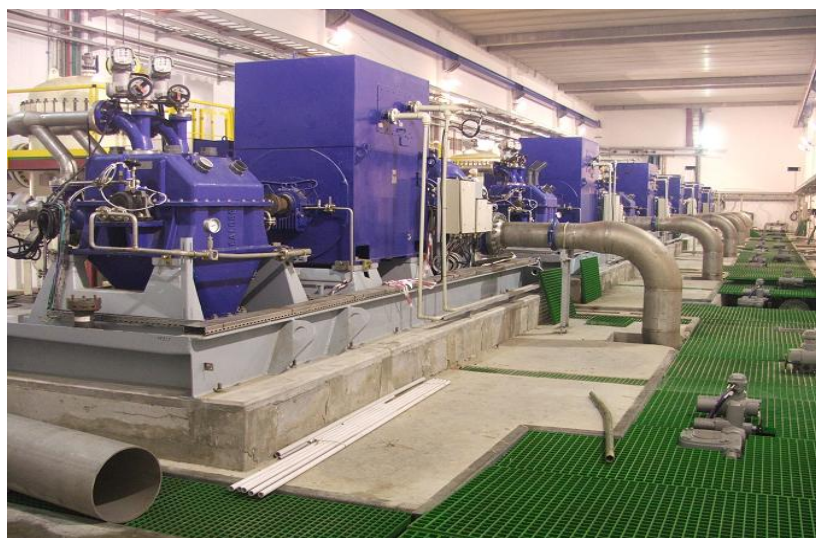
Figure 2 A– Palmachim train include ERT+MOTOR+HPP
