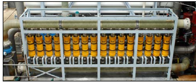
Figure 1: PX device array serving one SWRO train.
