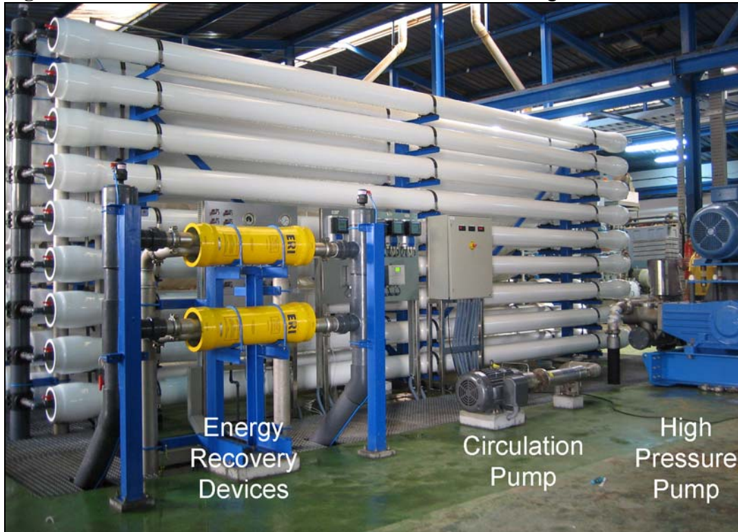
Figure 3. Seawater SWRO Process with PX Pressure Exchanger ERDs.
