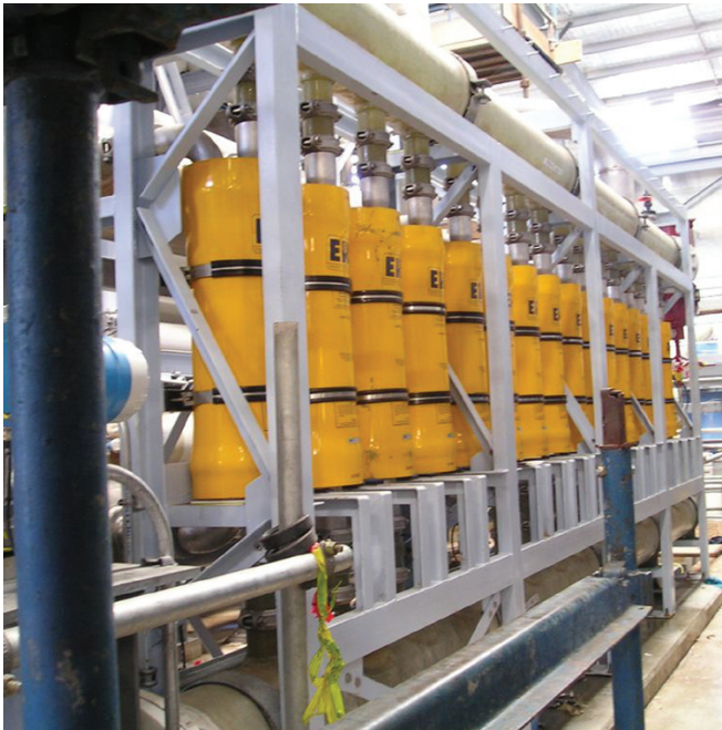
Figure 5. Perth, Australia 144,000 m 3 /day desalination plant (train #1)
