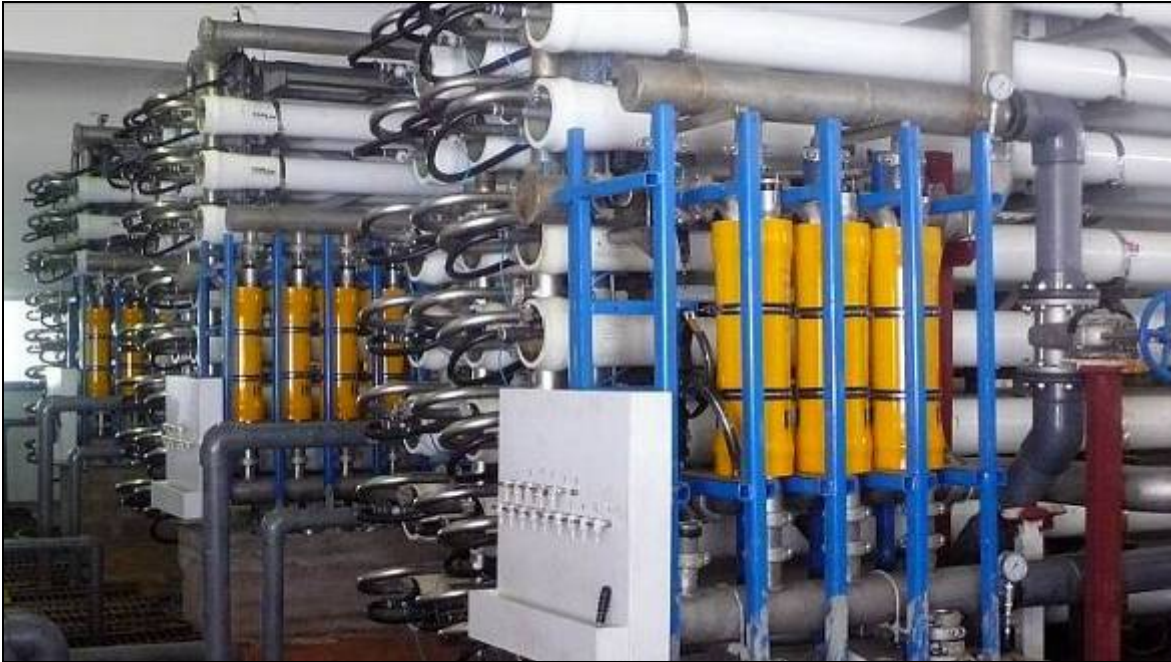
Figure 7 – Three PX Arrays at the Newieba Plant
