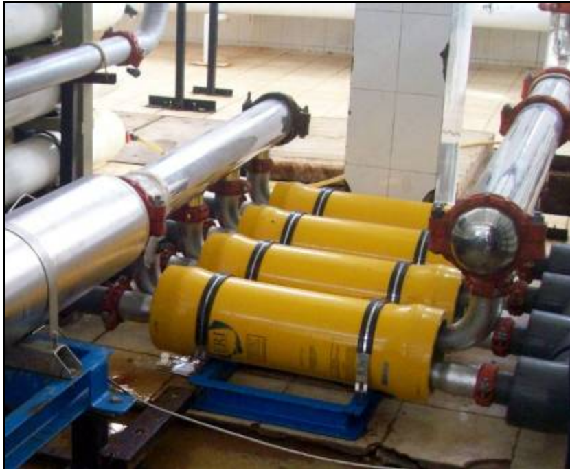
Figure 8 – PX Device Installation at the Sina Plant
