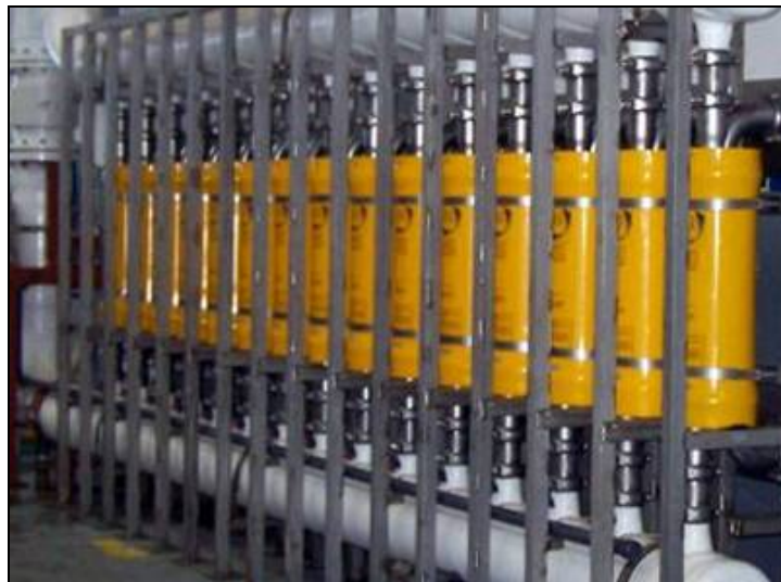
Figure 6 – PX Installation in the Las Palmas III Plant
