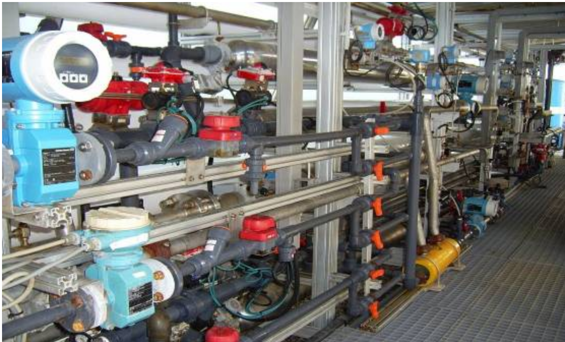
Figure 4 – The SWRO Process at the Tordera Pilot Plant
