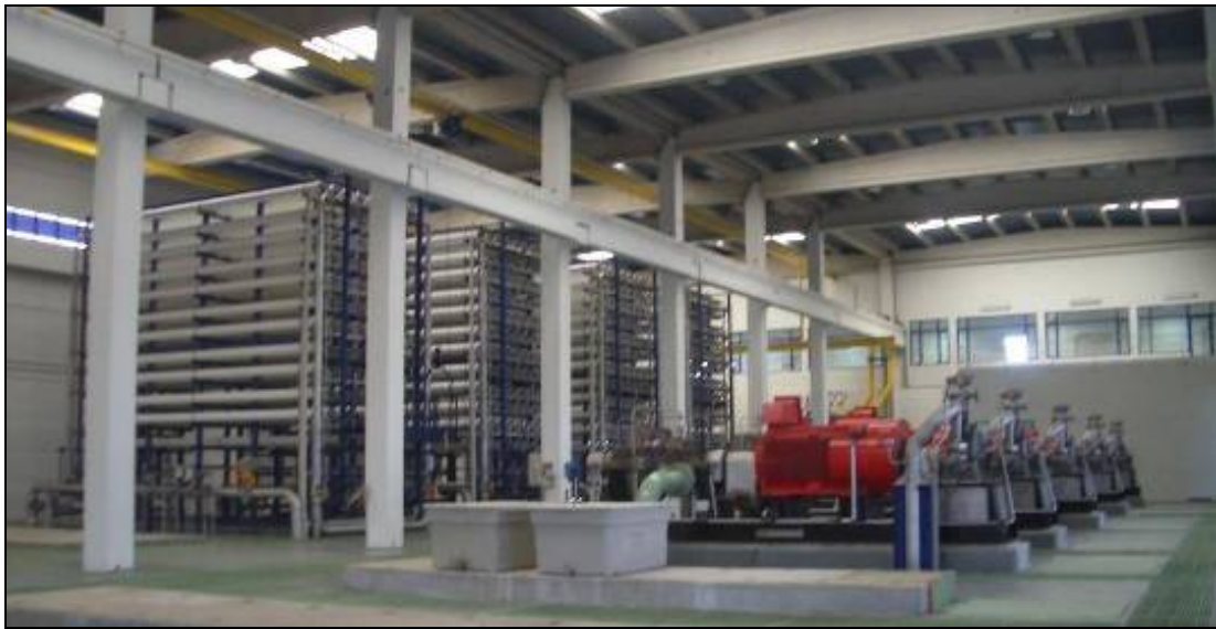
Figure 6 – The Legacy Design of the Tordera Plant
