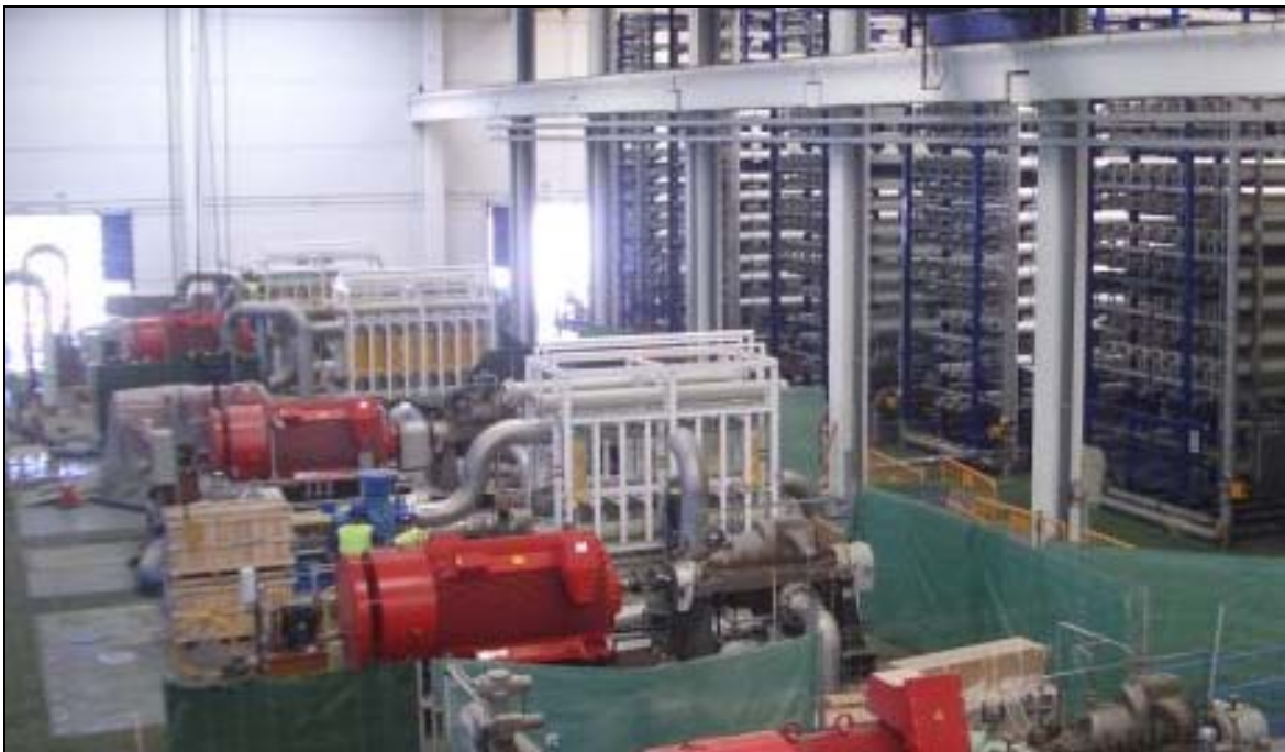
Figure 7 – SWRO Section of the Plant after Retrofit
