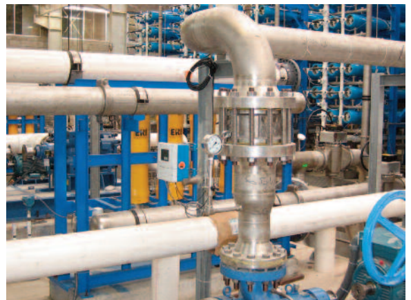
The plant is the largest in Mexico and provides municipal drinking water to approximately 40,000 local residents
