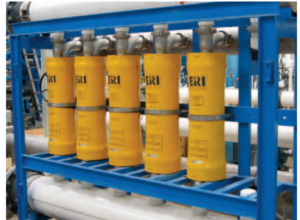
One of four PX Pressure Exchanger trains with provision for a sixth PX for future expansion
