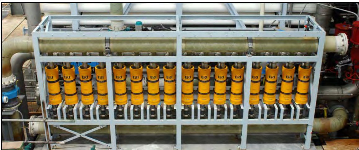
Figure 3 – PX Device Array Serving SWRO Train 6A
