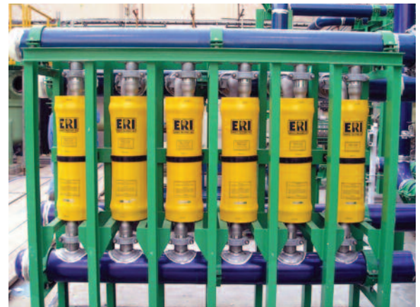
FEWA, UAE, 5,000 m 3 /day Modular Rack Assembly
