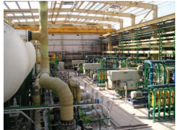
FEWA, UAE, Ghalilah Desalination Plant (Phase I/II) 14,700 m 3 /day
