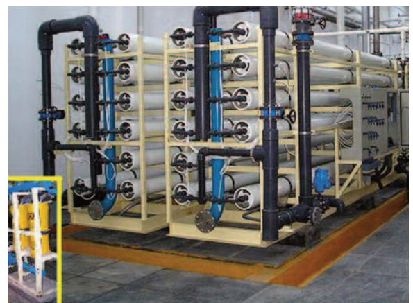
Membranes and Pressure Exchanger Devices
