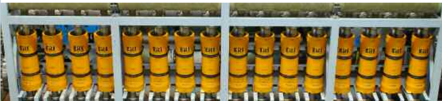
Perth SWRO Plant - Water Corporation - Kwinana, WA, Australia | Capacity: 144,000 m 3 /day
